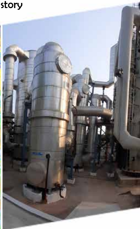
2000 TPD Sulphuric Acid Plant, 2x350 TPD Phos Acid Evaporator & FRU Coromandel International Ltd., Kakinada Design and Construction Stage.
